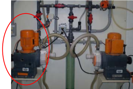
New Prominent Sodium Hypochlorite Pump
