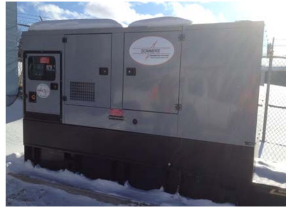
New 150 KW Generator Set
